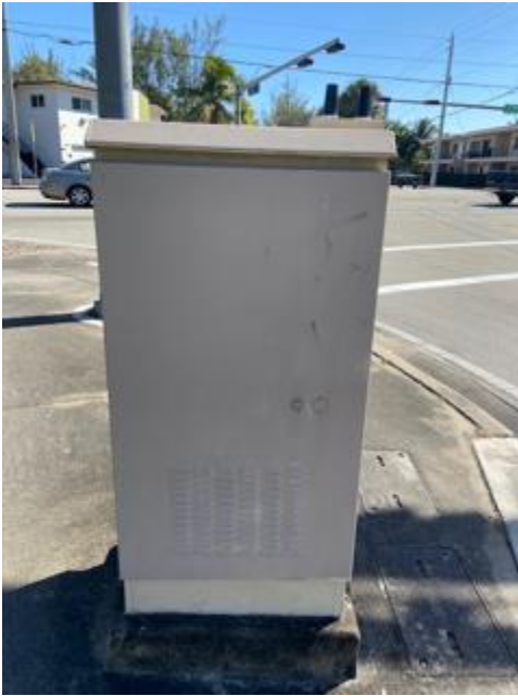
Utility Box (sidewalk)
