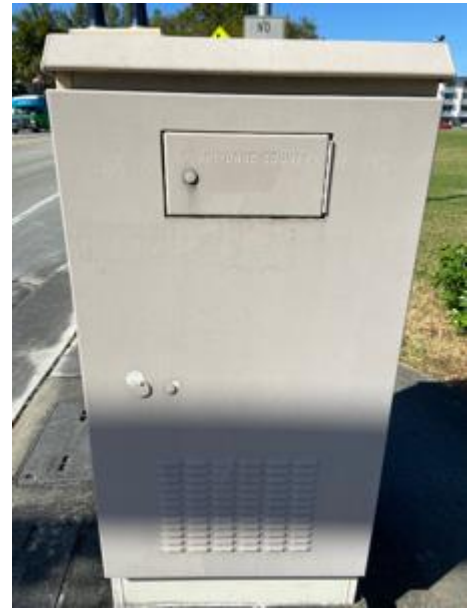
Utility Box Side 3
