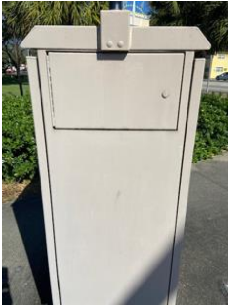
Utility Box Side 2
