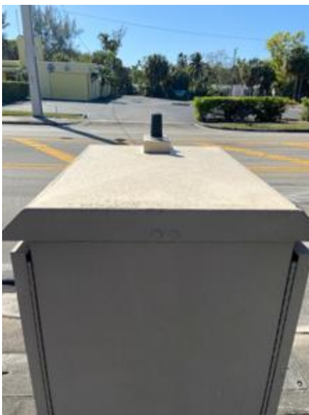
Utility Box Top View/Antenna
