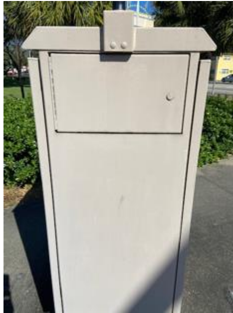
Utility Box Side 2
