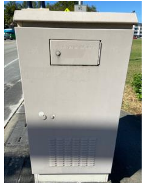
Utility Box Side 3
