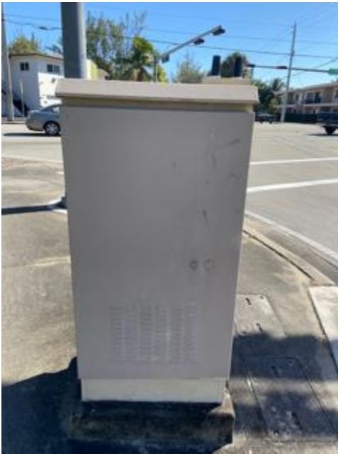
Utility Box (sidewalk)
